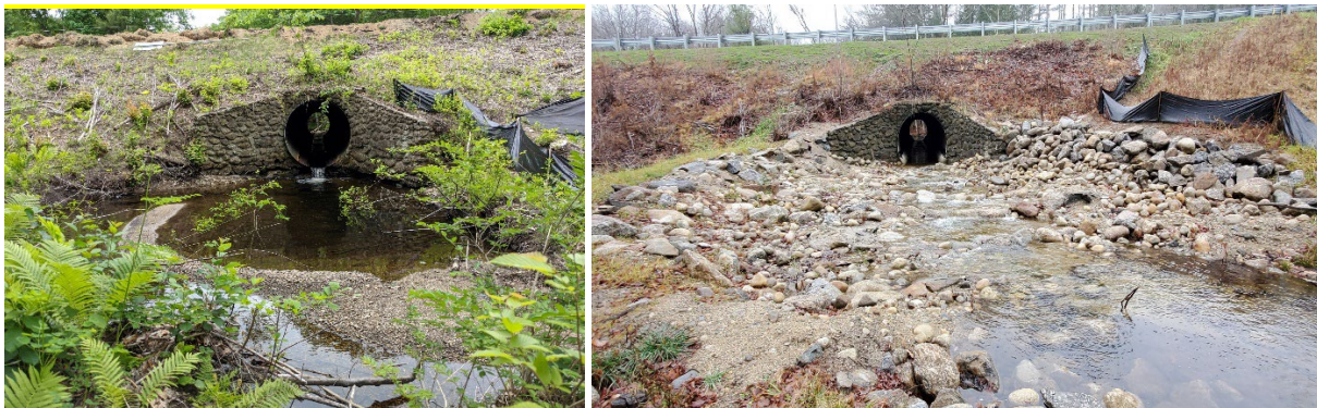
Figure 15. Perched culvert (left) and same culvert with a rock ramp (right).
