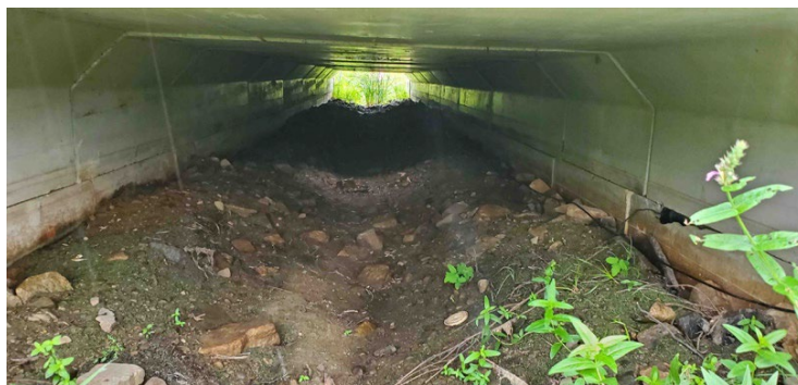
Figure 16. Dedicated turtle crossing structure.
